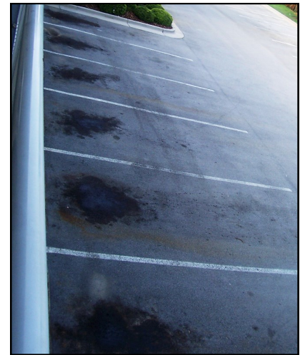
Typical damage from deterioration is caused by substances such as oil. Without sealcoat's protection, the oil is able to corrode the pavement.
