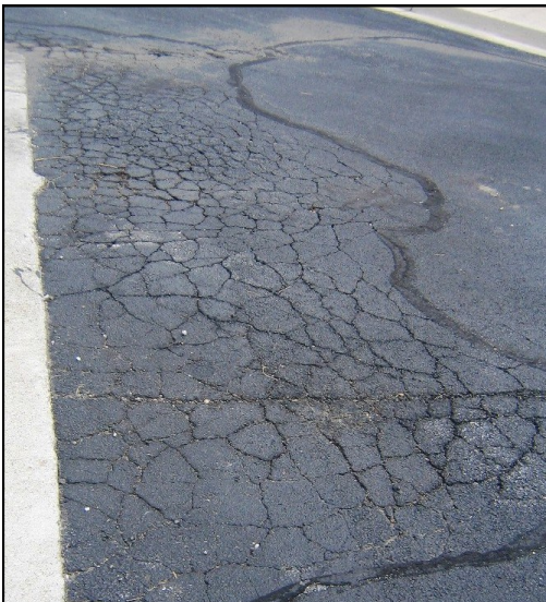
Alligatoring pavement, or an interconnected area of cracks, lead to serious pothole and liability issues that must be repaired at full depth.
